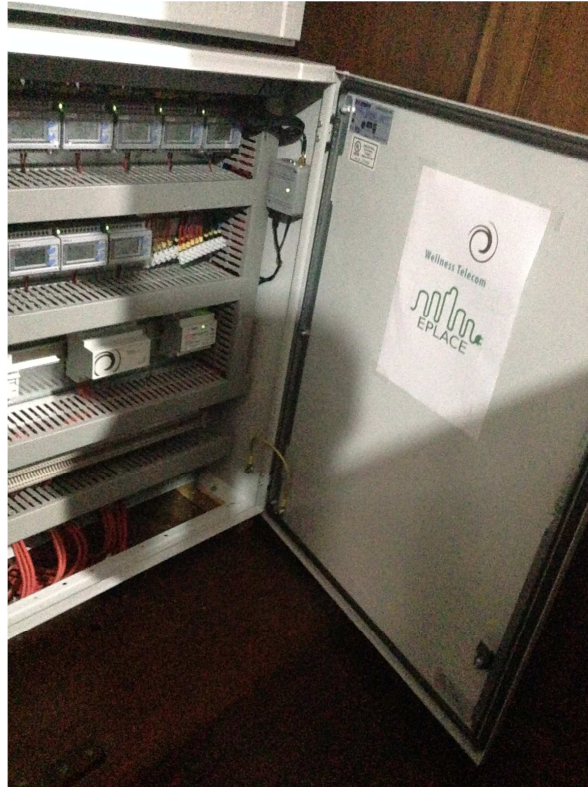
Figure 1: WeSave installation in City council of Cartaya
